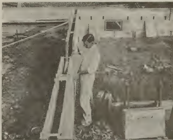
Constructing a double wall with concrete blocks. In this case the air space is continuous and furring the interior is unnecessary
